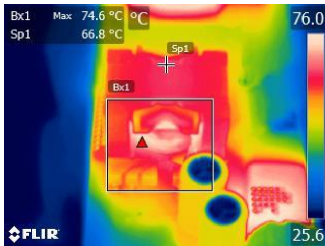
Figure 32 – Bx1 – DCDC Main Transformer (T3 Wire). Sp1 – DCDC Main Transformer (T3 Core).
